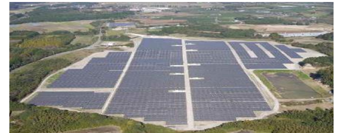
Kuma Nishikimachi Solar Power Plant External View
