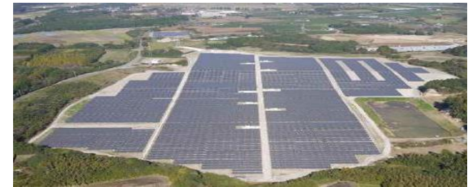
Kuma Nishikimachi Solar Power Plant External View
