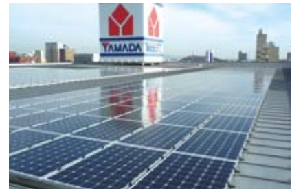
Solar power generation system installed on a store roof
